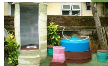
Biogas Toilet cost P 500,000.00 complete packages (basic training, installation, biogas stove and six months warranty)
